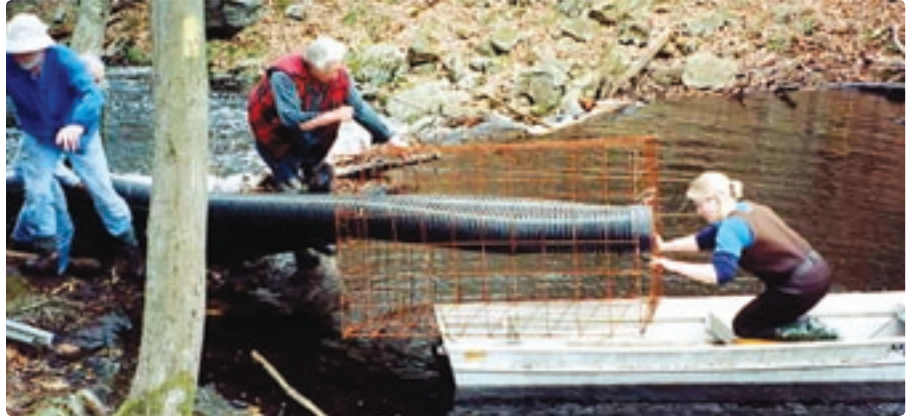
Becca DeWeerd and Skip Hilliker of The HSUS lower a beaver impeder into the water. The rectangular mesh "cage" around the pipe prevents beavers from plugging it up with debris, so water will continue to flow through the dam, and the nearby road will no longer flood. LAURA SIMON/THE HSUS
